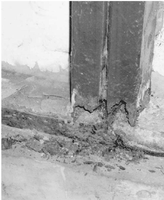
FIGURE 10.21 Bases of cold-formed wall studs supporting trusses in this early-vintage pre-engineered building are completely corroded from repeated saltwater entry.
