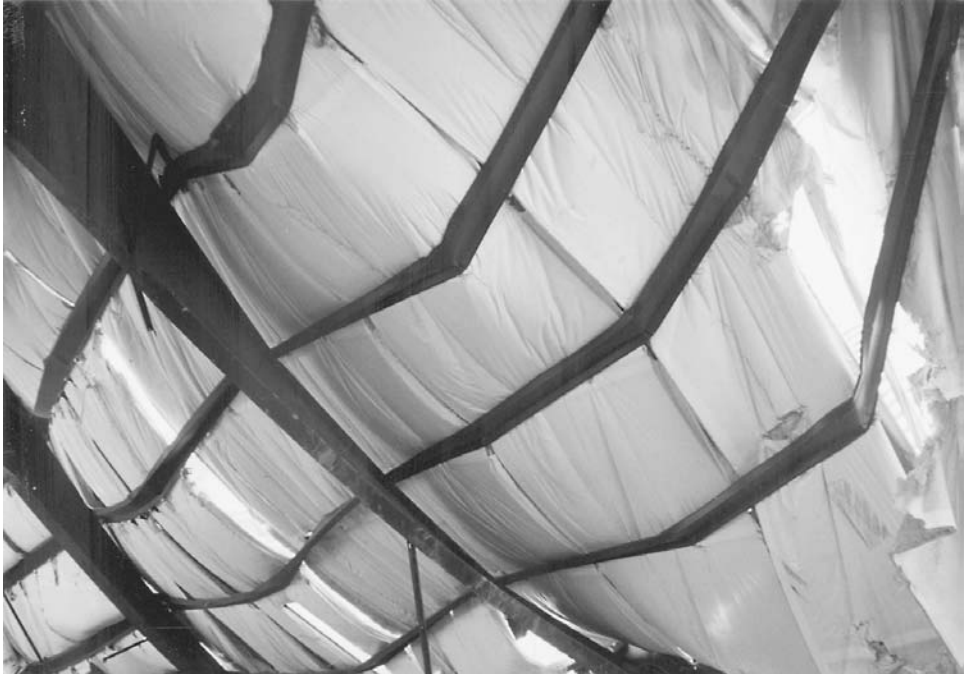
FIGURE 10.16 Building collapse under heavy snow accumulation.
