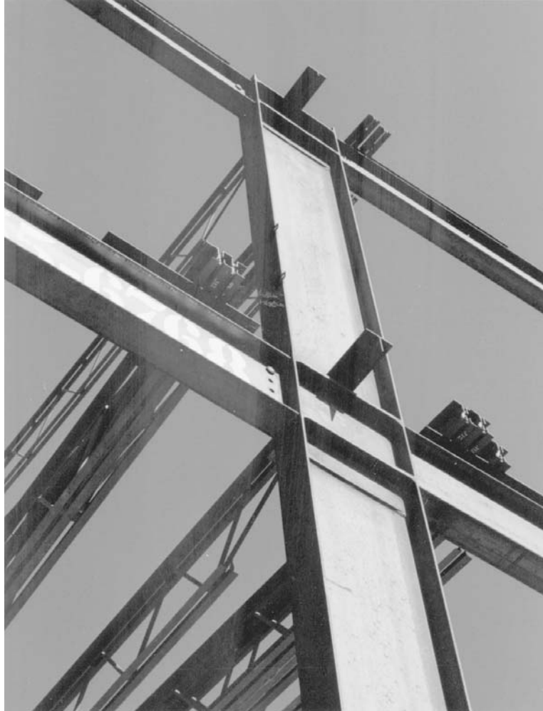
FIGURE 13.13 Details of exterior rigid frame shown in Fig. 13.12. ( HCI Building Systems, Inc. )
