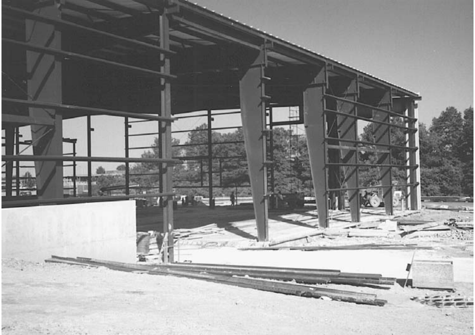
FIGURE 16.9 The roof of this pre-engineered building is installed before the walls. (Photo: Maguire Group Inc.)
