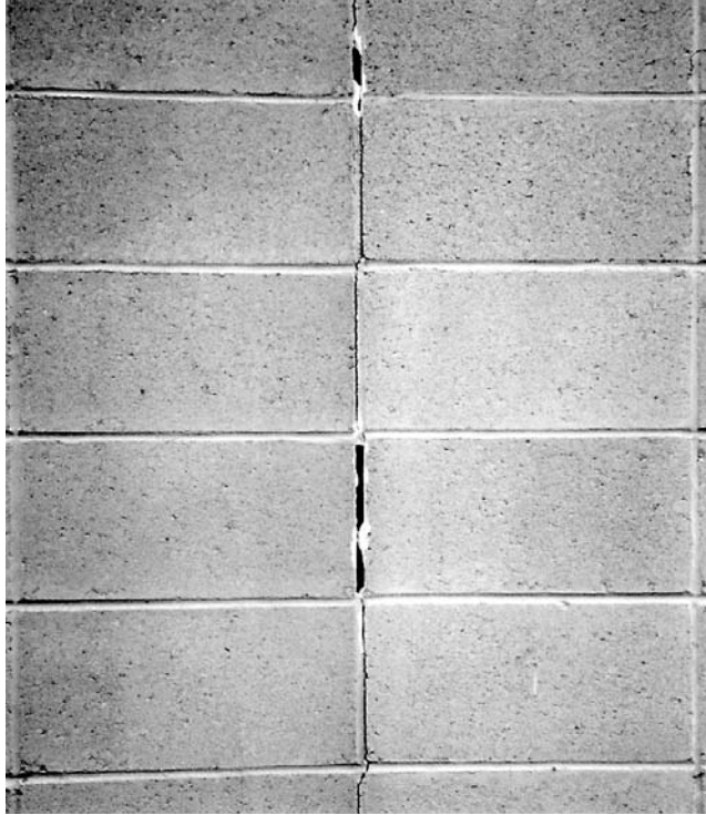
FIGURE 7.25 Watertightness of this single-layer stack-bond CMU wall is compromised by missing mortar. Daylight can be seen through the head joints.
