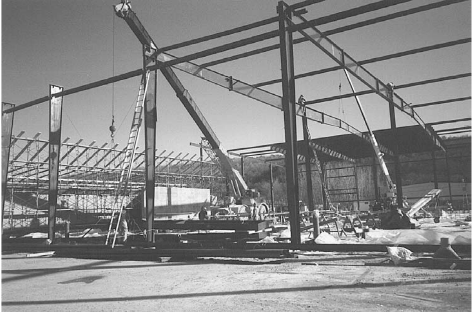
FIGURE 16.1 Assembly of multiple-span rigid frames. The columns at left are stabilized by diagonal bracing and wall girts. (Photo: Maguire Group Inc.)
