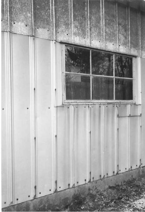
FIGURE 7.11 Rusted screws in through-fastened wall panels.
