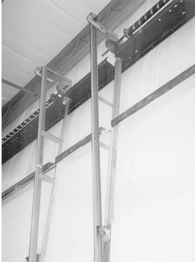
FIGURE 10.9 These overhead door jambs are not supported at the top by anything other than the girts—which were cut to allow for the jamb installation.
