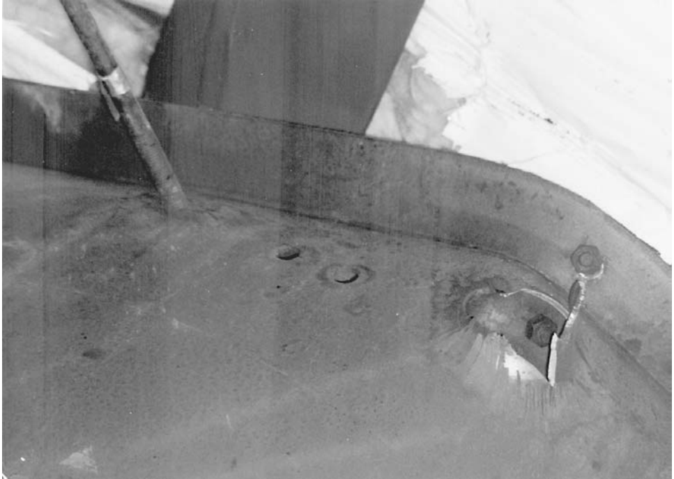
FIGURE 3.21 Fracture of the rafter web at the point of horizontal rod attachment. Note that the force applied by the bracing has also laterally displaced the rafter section.
