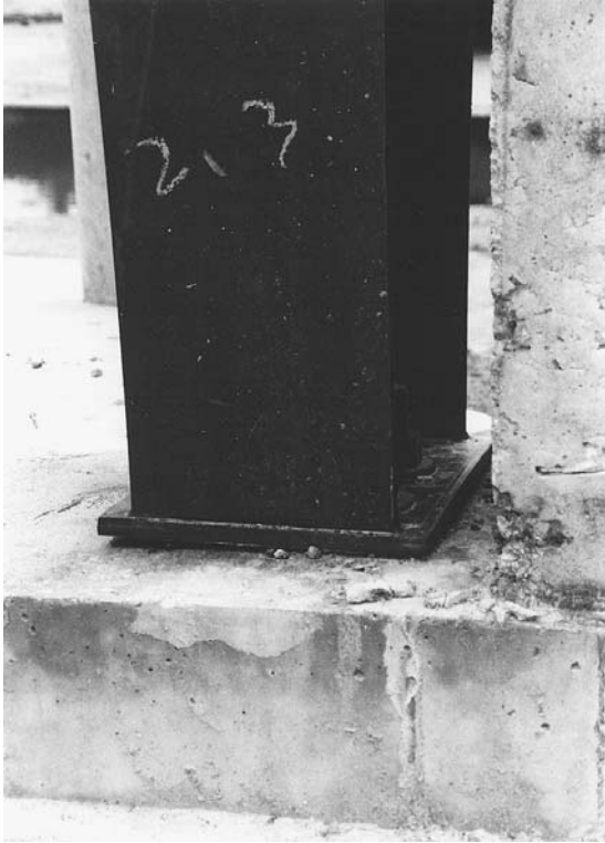
FIGURE 16.10 A gap under the column base plate.
