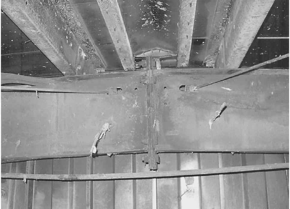
FIGURE 10.22 Effects of small fire on metal building system. The area at left is amplified in Fig. 10.23. Note also the method of rod attachment to frame. (Photo: Chabot Engineering.)
