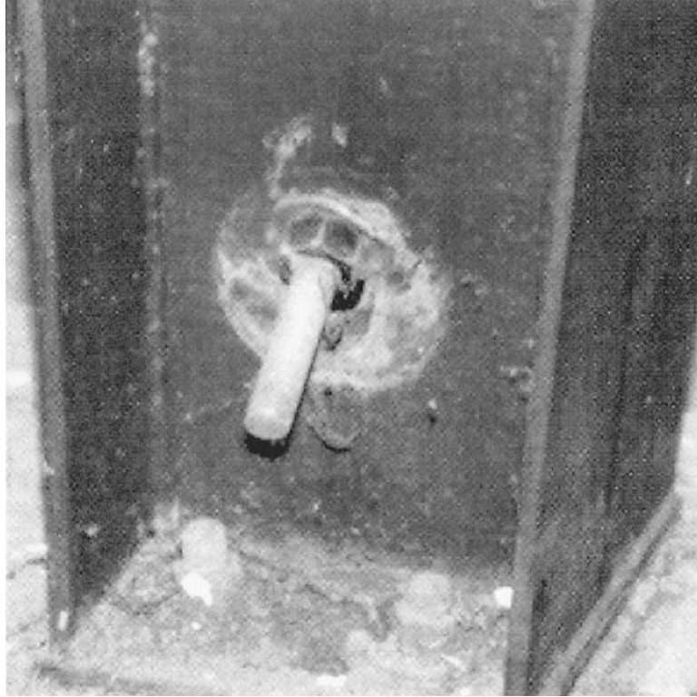
FIGURE 3.15 This is where a hillside washer was before the Northridge earthquake. ( J. R. Miller & Associates. )
