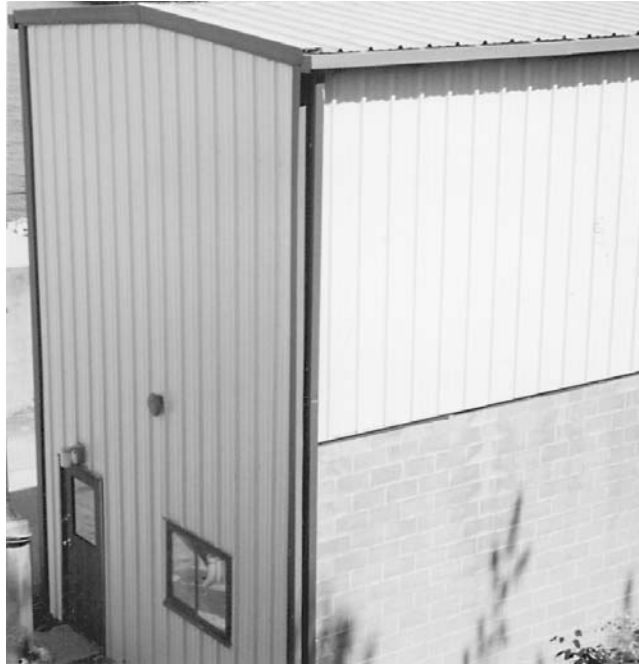
FIGURE 7.32 This partial-height CMU wall faces a hill and provides a measure of protection against rolling rocks and sliding debris.
