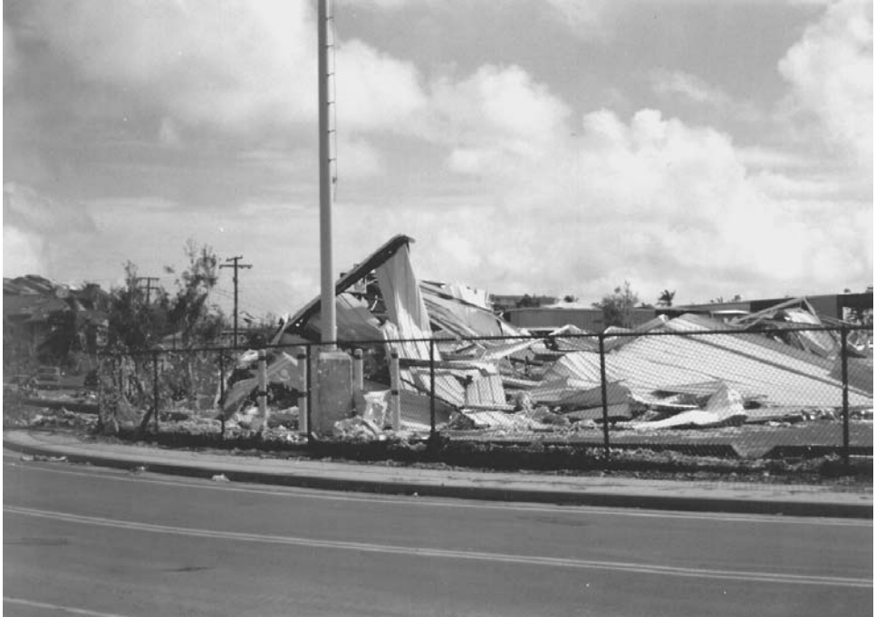
FIGURE 10.20 Total collapse of a metal building. (Photo: Structural Engineers Association of Hawaii.)
